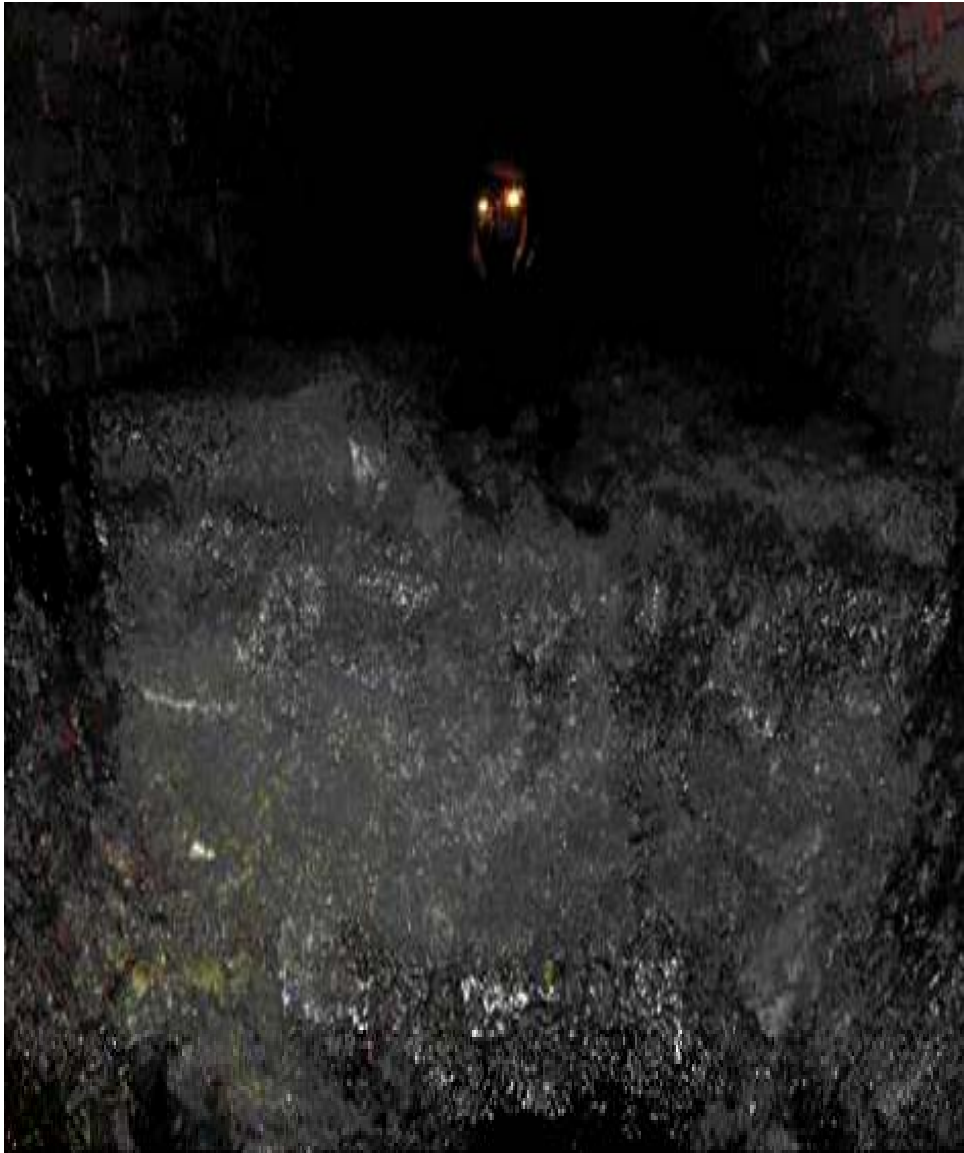
Condition of sewer before revamp
