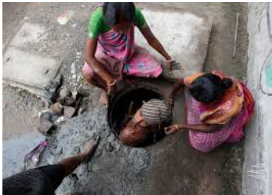
5. Drains gets CLOGGED
